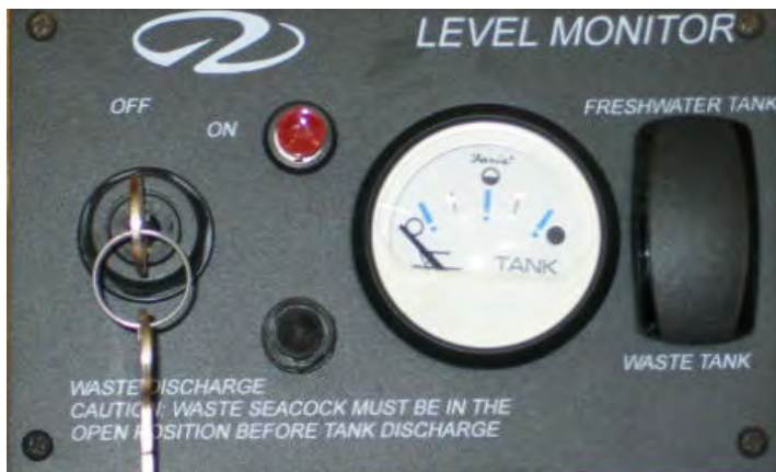
TYPICAL WATER/WASTE MONITOR PANEL
