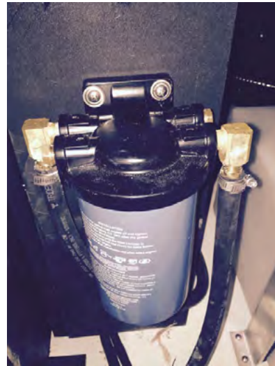
CHECKING IN-LINE WATER SEPARATOR FILTER
