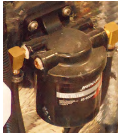
Generator In-Line Fuel Filter
