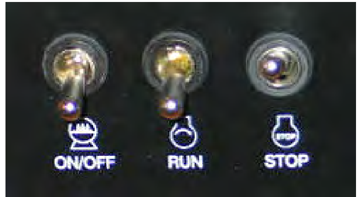
TYPICAL GEN-SET SWITCH CLUSTER- MAIN PANEL
