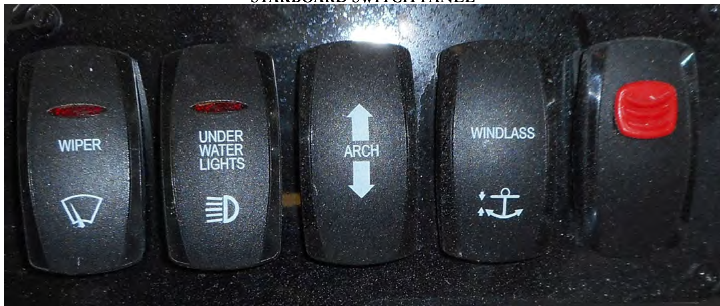
STARBOARD SWITCH PANEL
