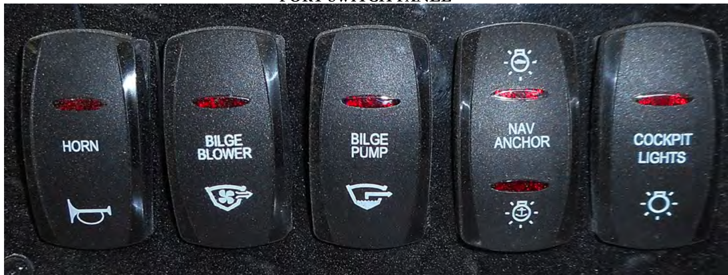
PORT SWITCH PANEL
