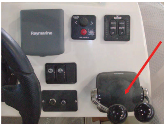
Wheelhouse Flying bridge
