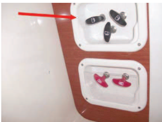
Remote pull switches - Supply tanks + generator
