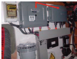
Location: Cockpit locker
