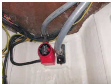
Electric bilge pump 12V - Engine compartment
